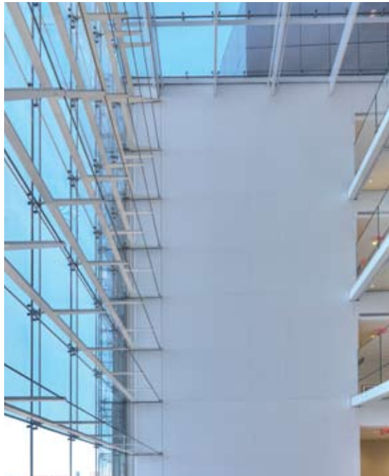
Interior view of atrium wall supported by a series of horizontal steel and cable trusses to take both wind and dead load
