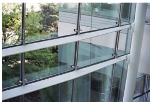
Horizontal painted steel plate beams resist wind load from the glazing and transfer it to the vertical steel jambs.
